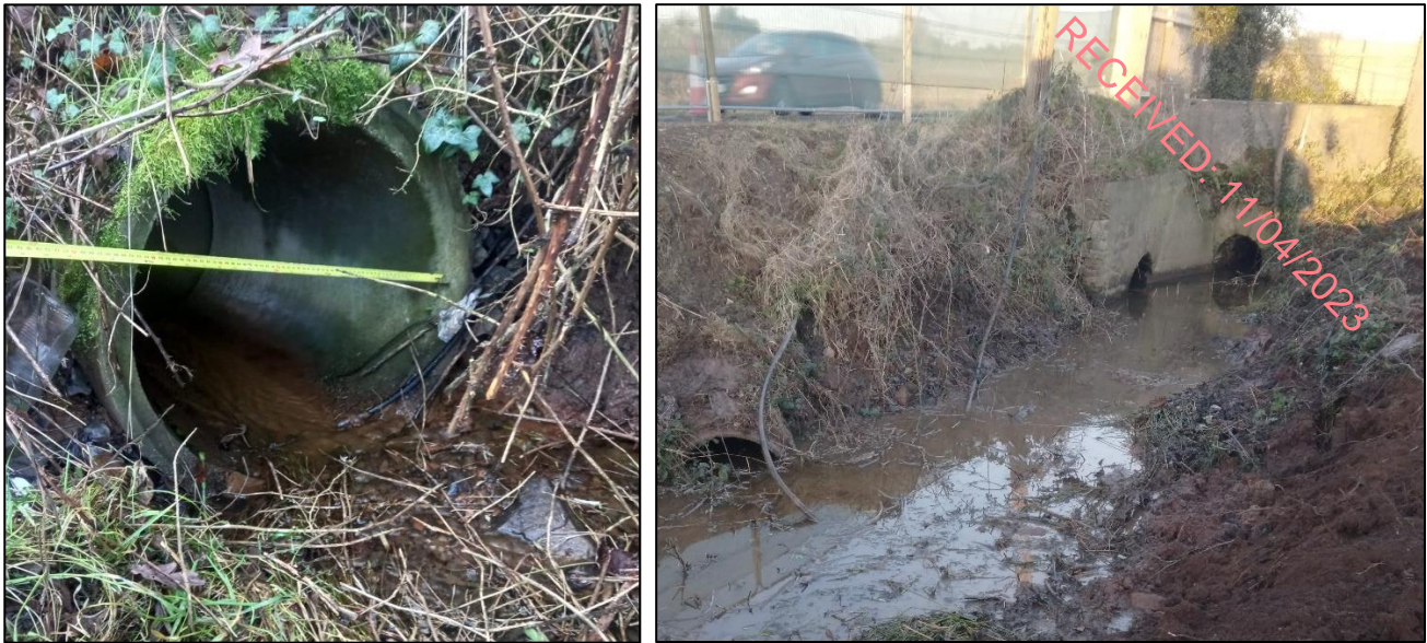
Figure 7: 750mm diameter culvert – North Entry on left and South Exit on right
